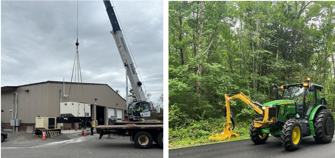
New Generator and Roadside Mower.
