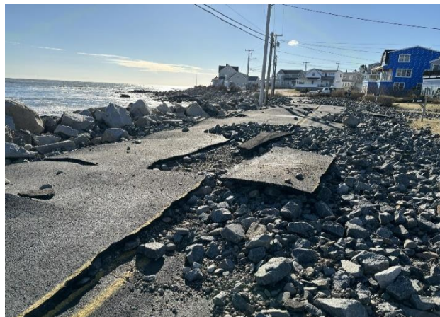
Storm damage from January and April 2024 storms.
