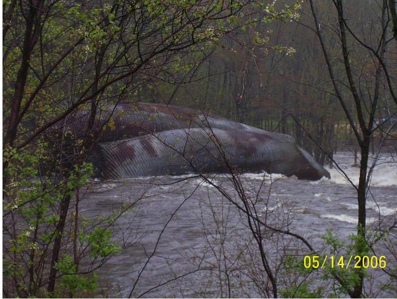
Captain Thomas Road Culverts Washed Downstream
