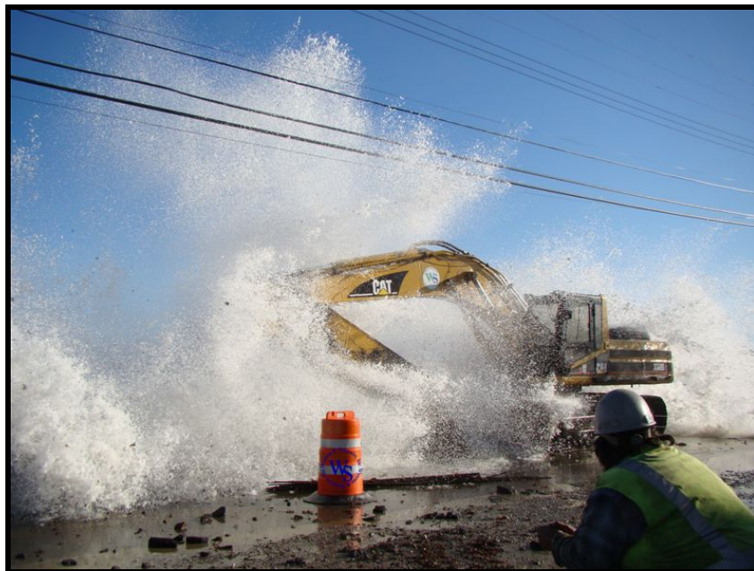
Splashover at Webhannet Seawall
